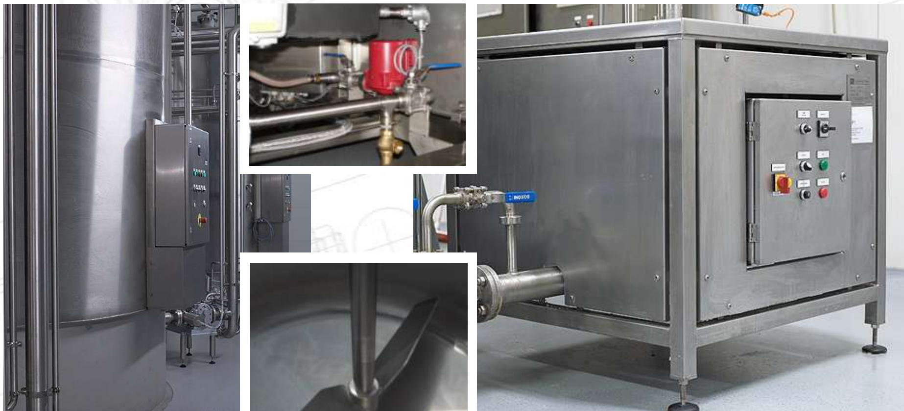
Storage- and melting tanks with agitator
